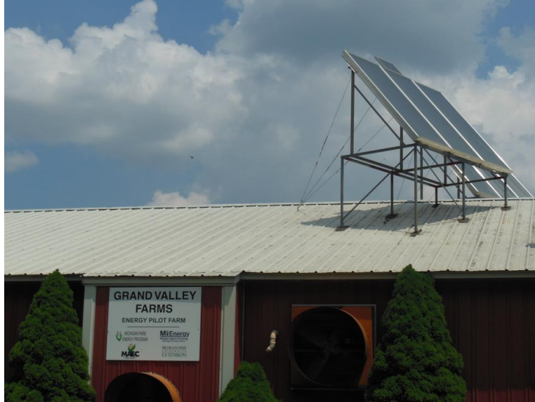
Figure 1: Solar Panel Placement
