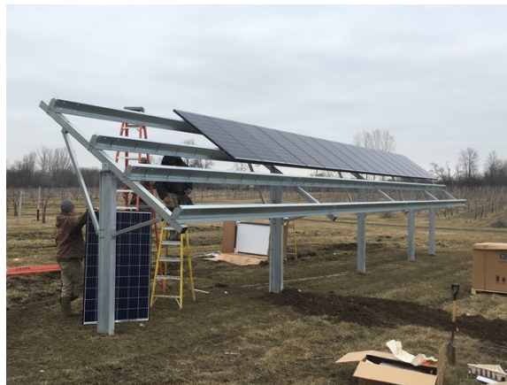
Harvest Energy during the installation process of the panels located at Plymouth Orchards.
